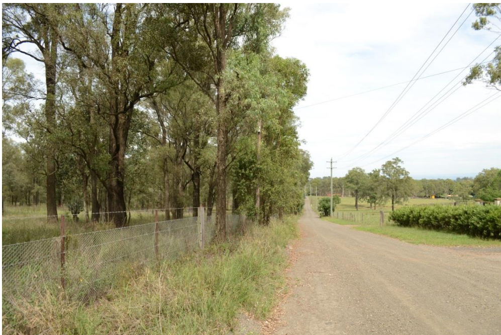
Figure 10 Example of an overhead transmission line
