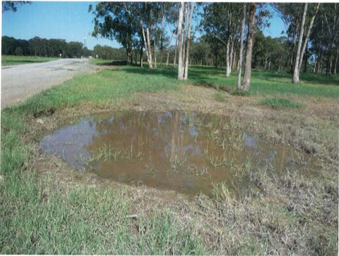
P 2 Access road east of Quarry. View east. Overland flow water emerging to pond south of the quarry access road.
