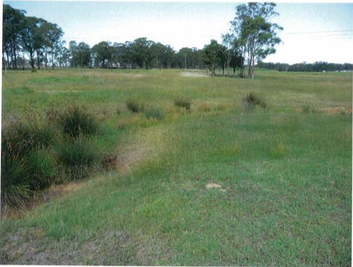
P4 Dispersive erosion on creek line, Fill area (GD5a) in background.
