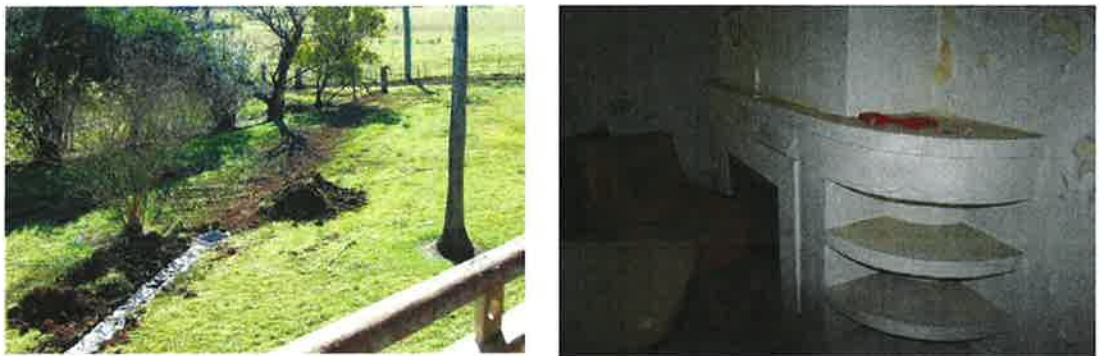
Figure 4.3 View of remedial drainage works (Heritech Consulting 2009) (left) and detail of fireplace with water damage to wallpaper (right)
