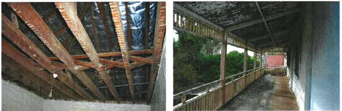
Figure 4.7 Detail of ceiling from second level (right) and view of upstairs verandah (right)
