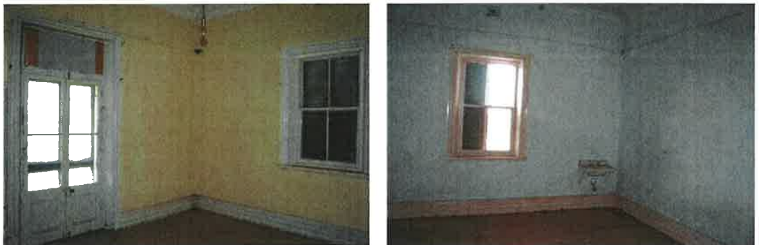
Figure 4.5 View of Upstairs rooms. Note the sink fitting in the corner of the figure on the right
