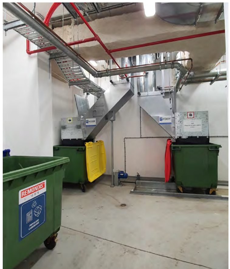
Fig 16.6.A Recycling in basement back-of-house
