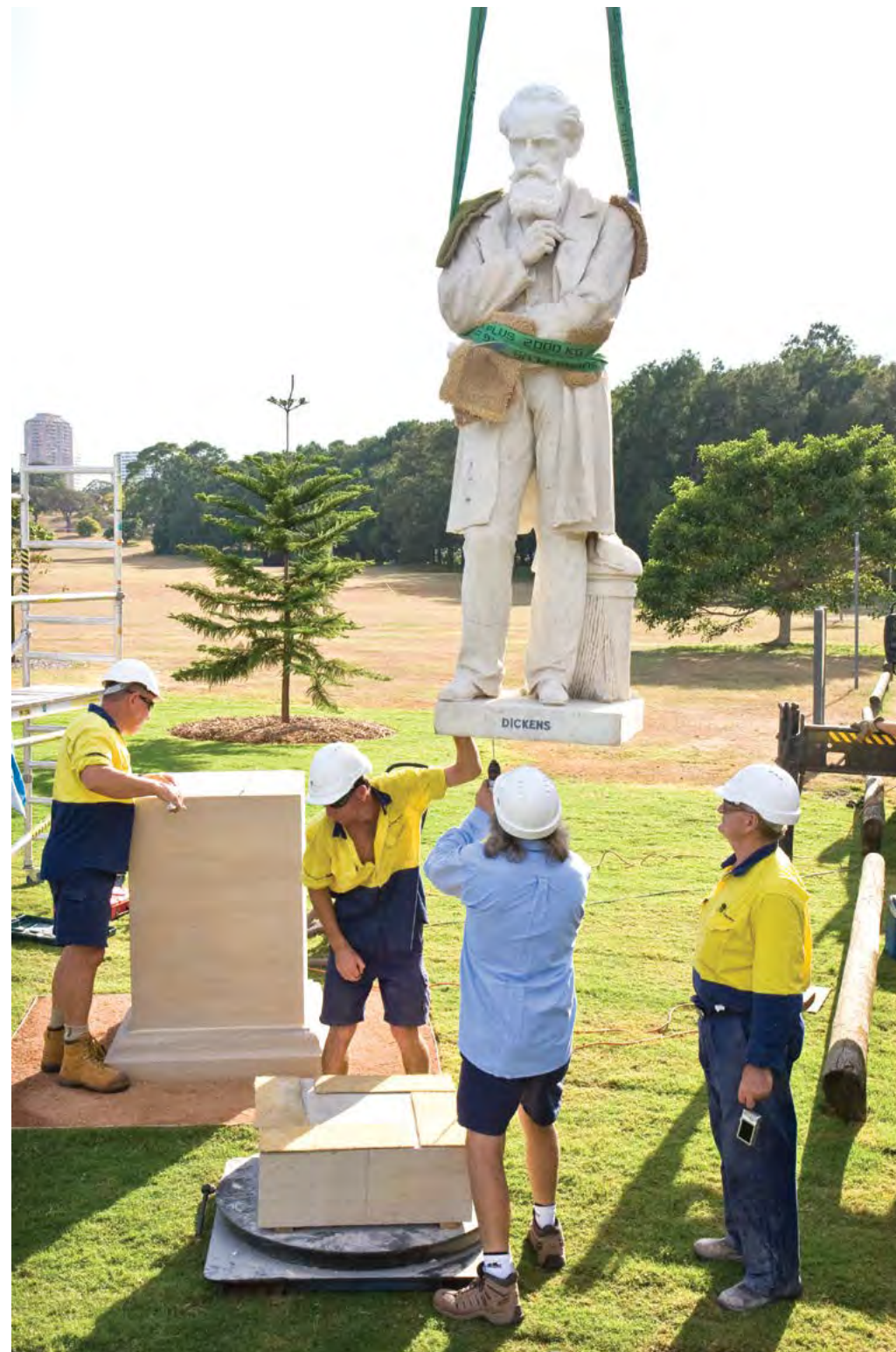
Installation of the statue in Dickens Drive, Centennial Park by stonemasons Luke Wijtes, Ben Gardener, Gary Rimmer and Reuben Varfi. Photograph by Michael Nicholson, 2011.
