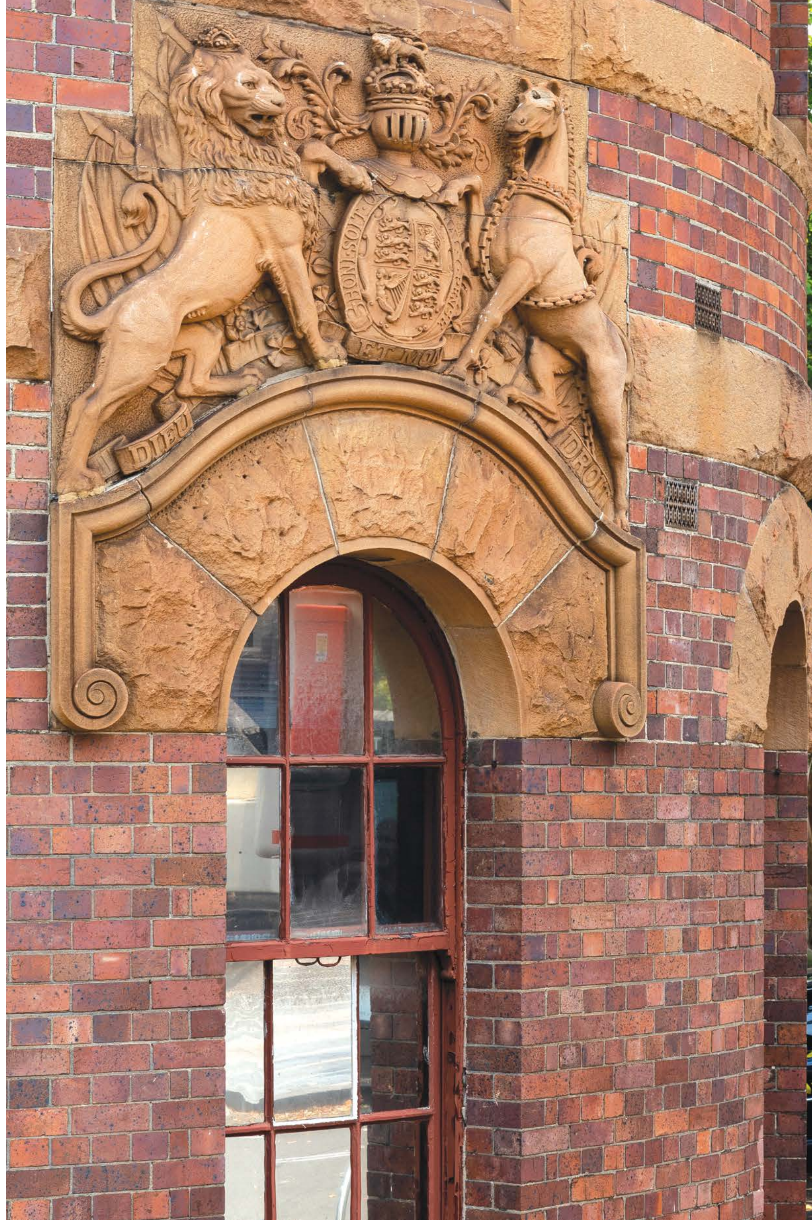
Right: Heritage architect Joy Singh and stonemason Ian Goulding inspect the facades of former Darlinghurst Police Station. Photograph by Douglas Frost, 2019.
