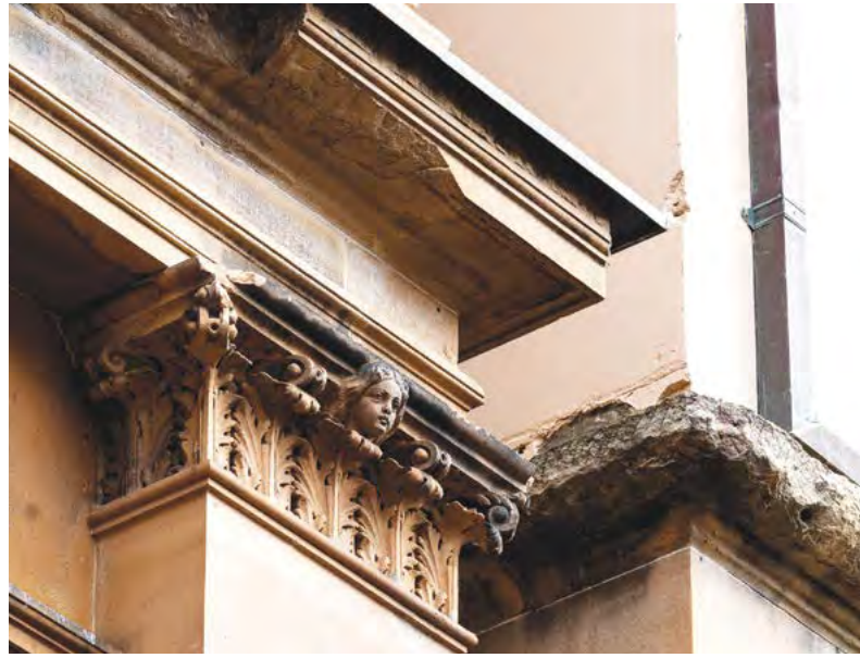
Above: The Sydney Hospital façade features typical cornice deterioration patterns. Damp conditions result in black staining, biological growth, erosion and cracking. Photograph by Douglas Frost, 2020.
