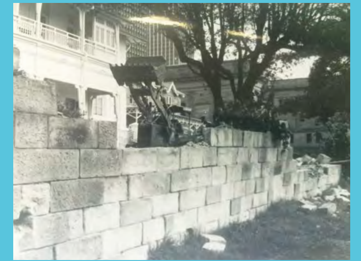
Mid 1970s demolition of the Macquarie era boundary wall, Hospital Road, just prior to the protection afforded by the NSW Heritage Act 1977.
