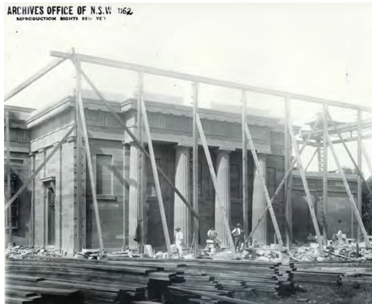
Darlinghurst Courthouse designed by Mortimer Lewis receives additional wings designed by James Barnet shown here in construction on January 1st 1885. Image shows a timber gantry crane for lifting stones. (State Archives and Records Authority of NSW).
