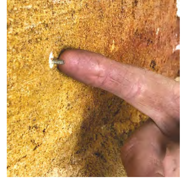
Above: Small stainless steel pins were installed to finish flush with the stone wall at Fort Denison. This provides objective information on the rate of surface loss over time to develop a cyclic desalination program. Photograph NSW Public Works.
