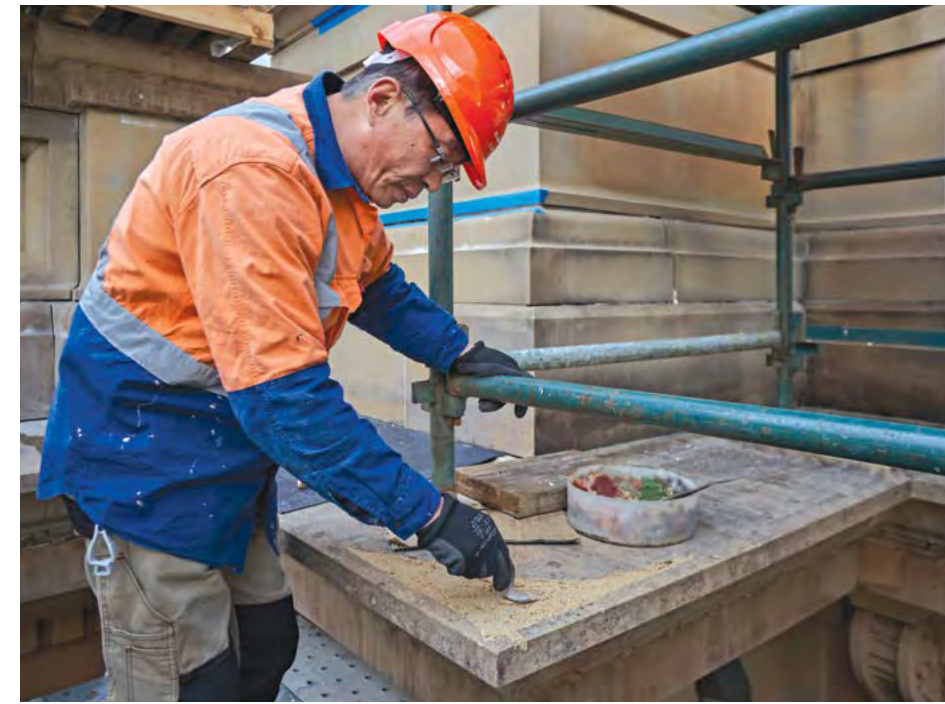
Right: At the Australian Museum, stonemason James Dong patches the top of a stone, rebuilding its water-shedding profile. Photograph by Michael Nicholson, 2020.
