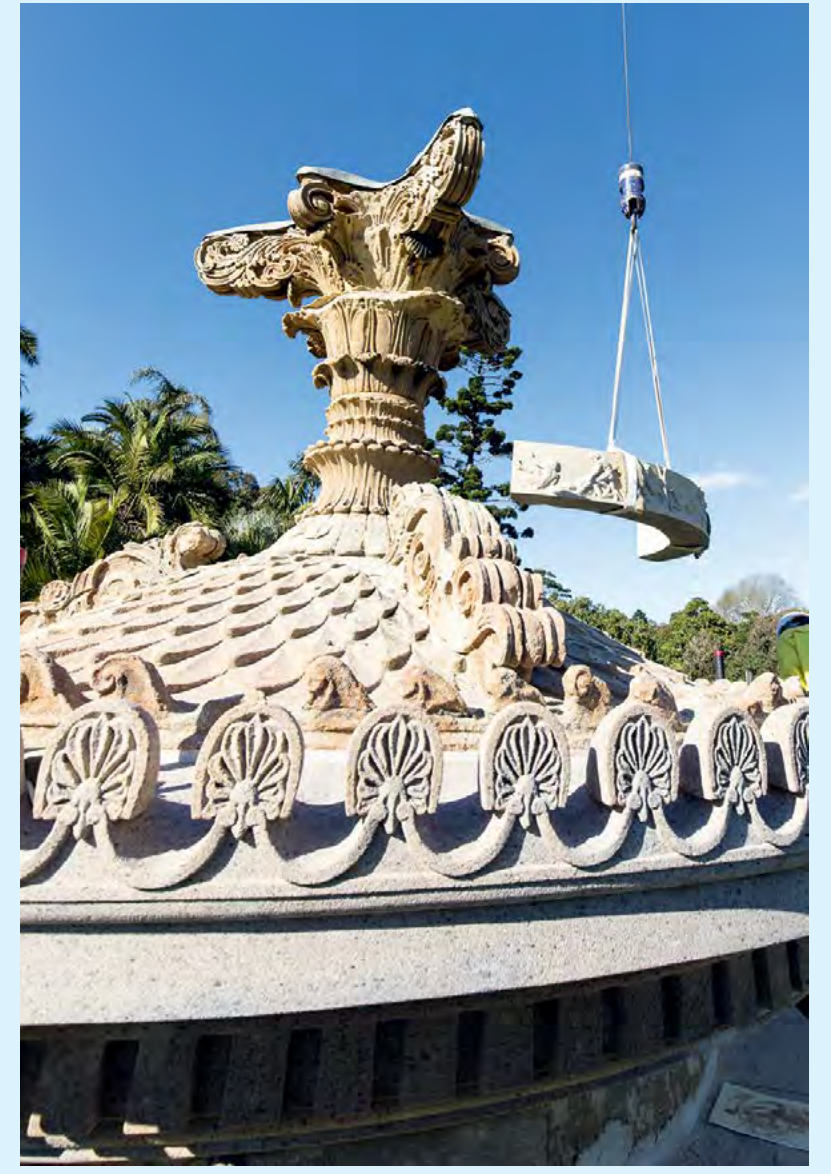
The recarved frieze stone being lifted into place, 2017. Photograph by Douglas Frost
