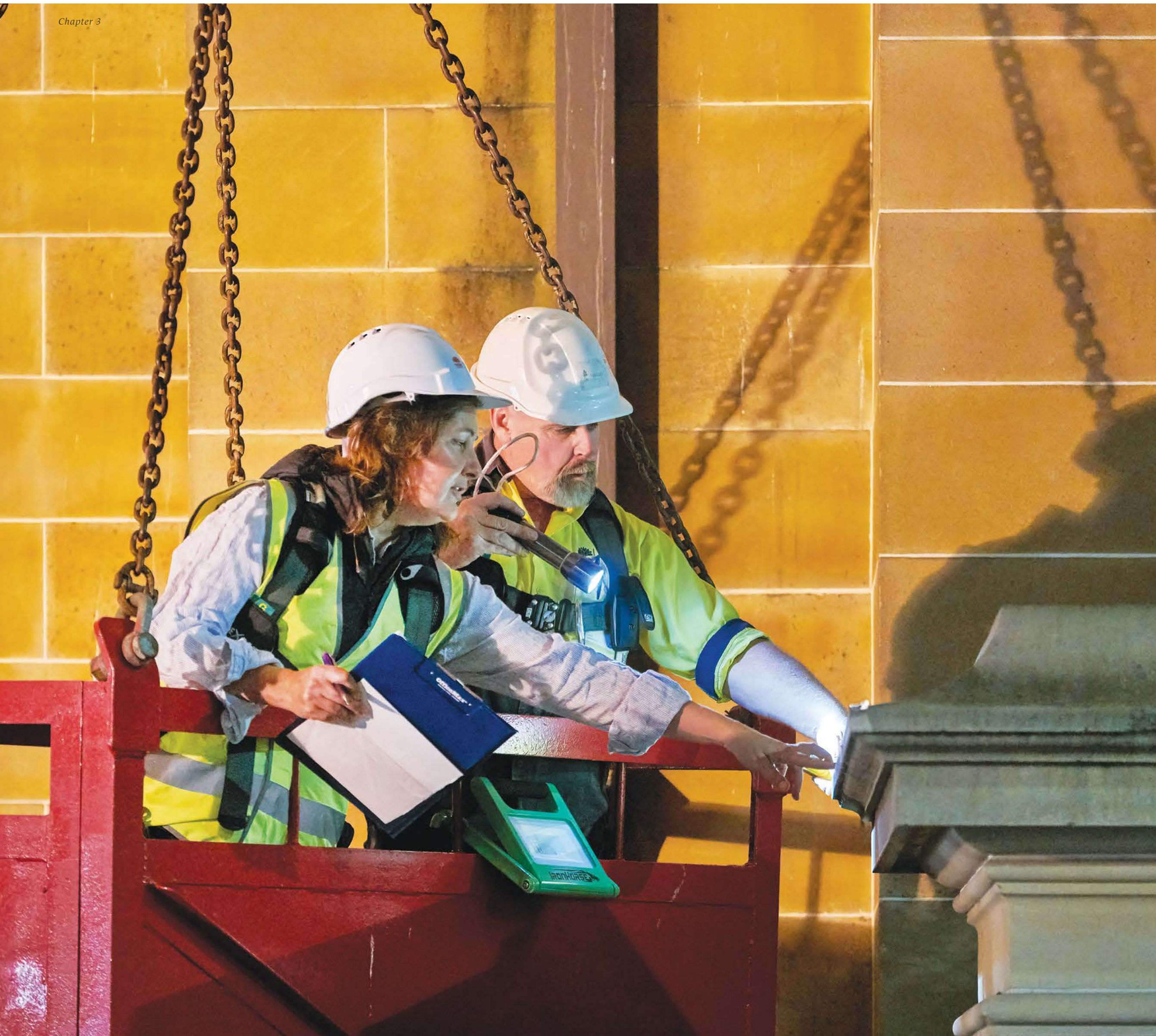
Left: NSW Public Works Principal Heritage Architect Kate Napier and Heritage Stoneworks' Senior Stonemason Craig Miller work through the night. They assess condition and scope repairs at close range from a crane box. Lichen and carbon build-up on exposed stones makes hairline cracks difficult to see at night, however lightrail track installation has prevented day time work. Stone is tapped to detect unsound stone, which is a safety risk in high level cornices overhanging publicly accessible areas. Photograph by Michael Nicholson, 2018.
