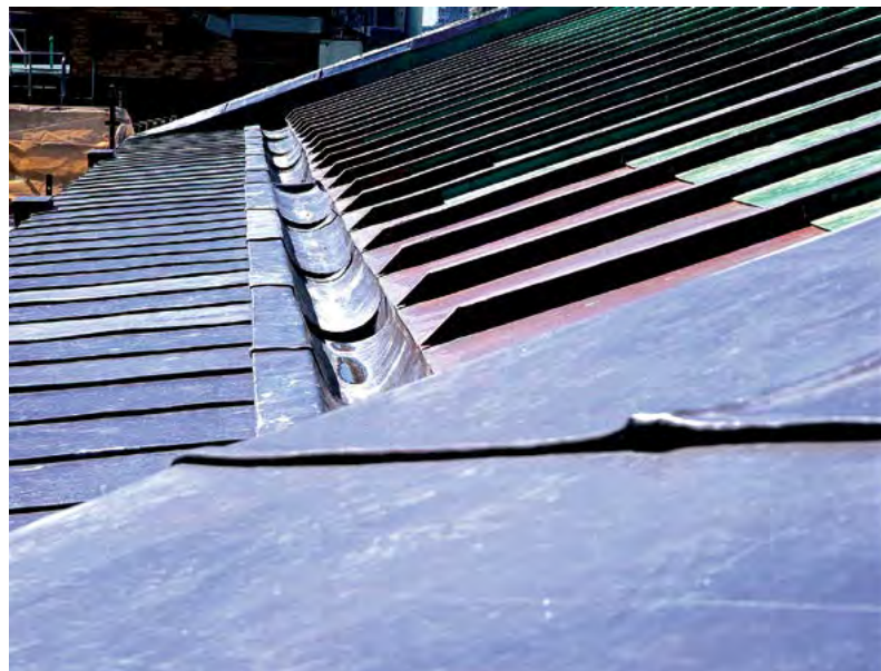
Below: Lead weatherings provide physical protection over the stone cornice and pediment of the Australian Museum. The Minister's Stonework Program has developed best practice lead detailing as a preservation measure to prolong the life of the stone. Photography by NSW Public Works, 2017.
