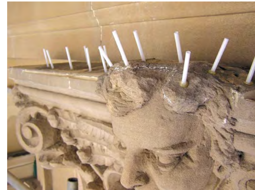
Right: Conservation of a carving sheltered under the overhanging cornice at Sydney Hospital. The cracked stone is stabilised by injecting a consolidating material to prolong the life of the stone.
